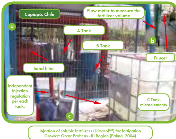
Figure 113. Injection of soluble fertilizers ( Ultrasol™ ) for fertigation. See details in photos a, b and c. Orchard "Cantera". Grower: Orcar Prohens, III Region, Copiapo Valley, Chile (Courtesy of growers, Picture took by Palma, 2004).
