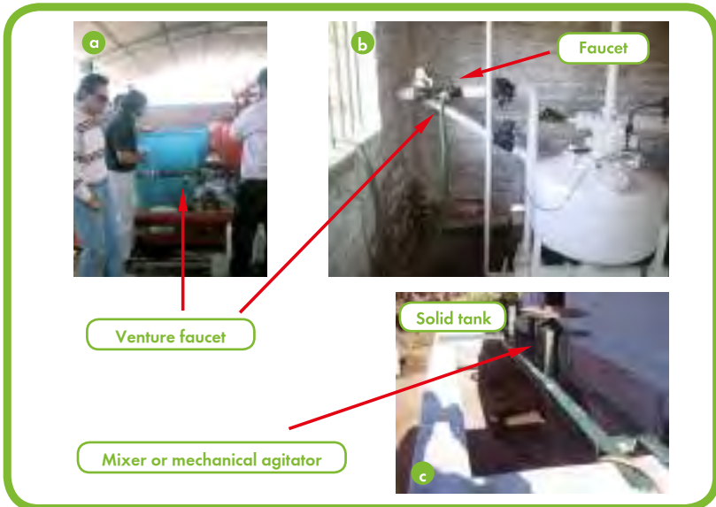
Figure 114. Injection of raw material fertilizers for fertigation in less sophisticated systems. Argentina and Chile (a, b and c) (Palma, 2004).
