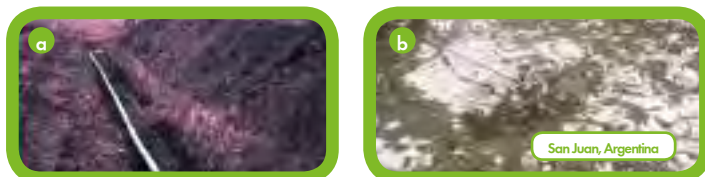
Figure 38. Installation of a drip irrigation system in Chile (a) and Argentina (b) (Ljubetic, 2003; Palma, 2003, Argentina).
